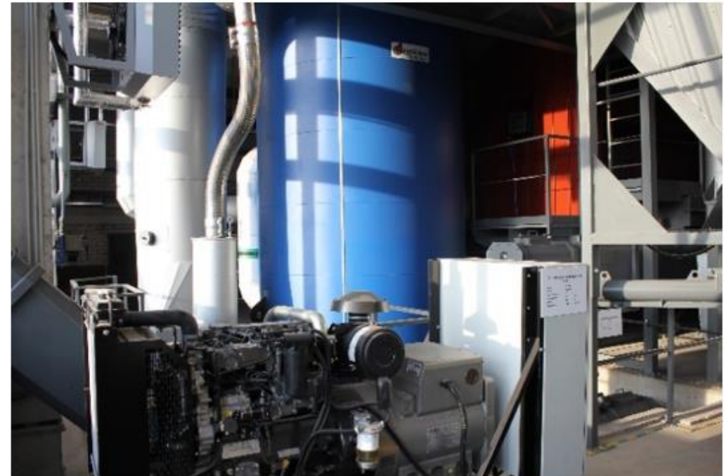
New biomass fired boiler
