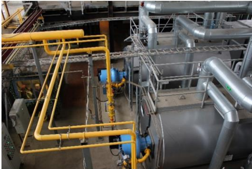
Old fossil fuel fired boiler
