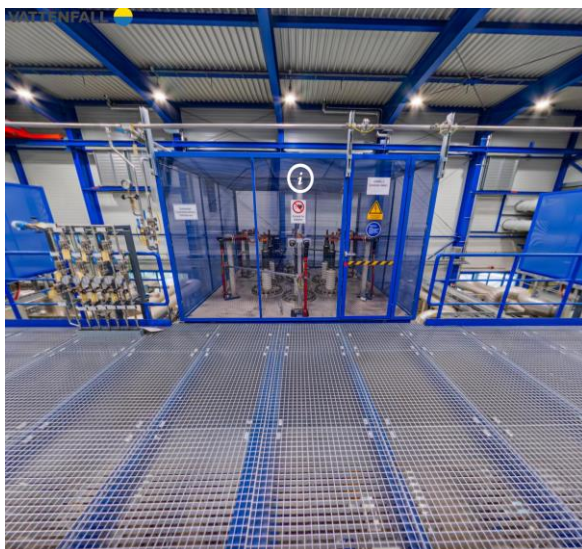
Image 42: Details on the P2H plant area
