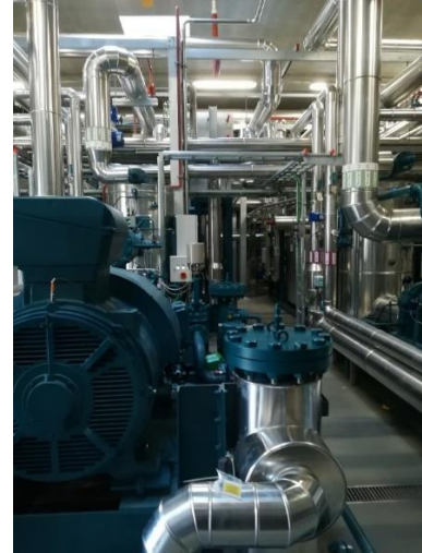
Image 27: Pumping station (Source: COWI)
