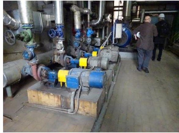
Image 8: Pumping station (Source: AGFW)
