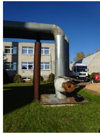
Image 4: Salcininkai boiler house
