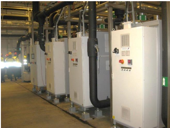
Image 24: Heat pumps system at MAX IV to produce hot water for the low temperature district heating network (Source: COWI)
