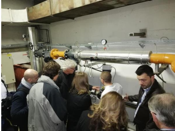
Image 13: Modernized substation of Tuzla DHS (Source: EPBiH)
