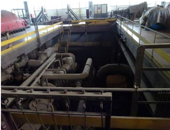
Image 9: Inside the main building of the CHP (Source: AGFW)
