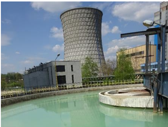
Image 11: Cooling tower (Source: AGFW)
