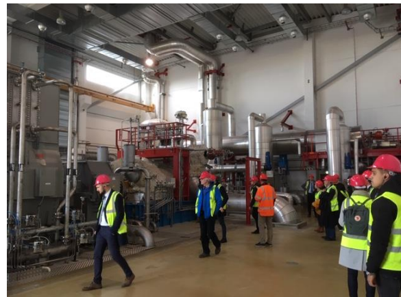
Image 21: Overview of the electricity production system at Örtofta power plant, showing also the steam pipes and other relevant installations (Source: COWI)
