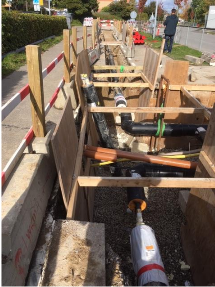
Image 33: Installation of the new pipes for the DH network in Østerby (Source: COWI)
