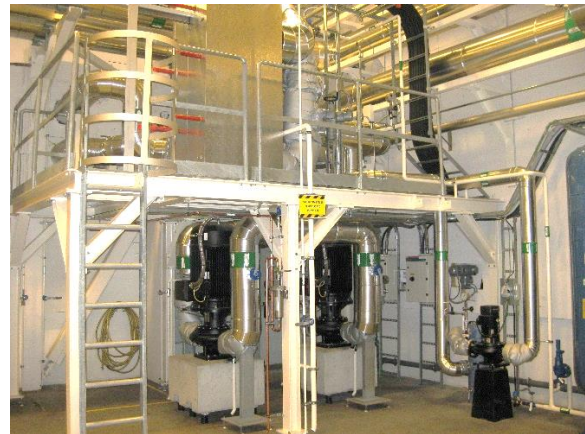
Image 25: Heat pumps system to produce hot water for the low temperature district heating network for Brunnsög (Source: COWI)
