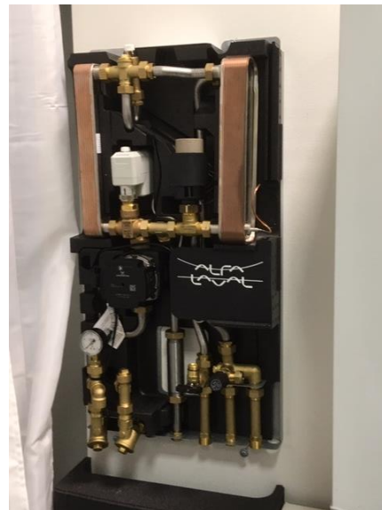
Image 32: Example of district heating unit equipped with two small heat exchangers, the first one for space heating supply and the second one for domestic hot water production (Source: COWI)
