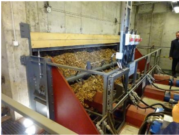
Image 3: Salcininkai boiler house
